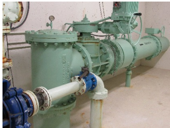
The big green 26 inch pipe is bringing in raw water from the wells.
