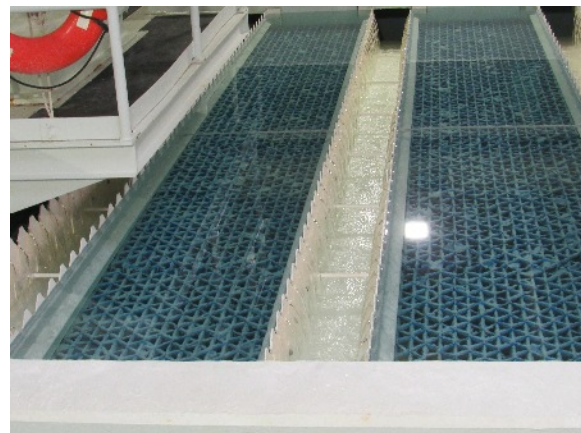
Some of the filtration system the water goes through before it is finished for use.
